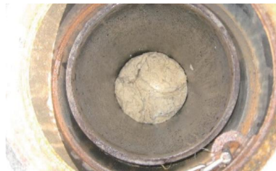
Oil deposit clogging
